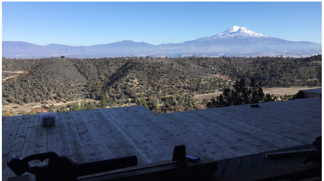
Photo taken from the platform of the cave toward the end of the restoration work.
